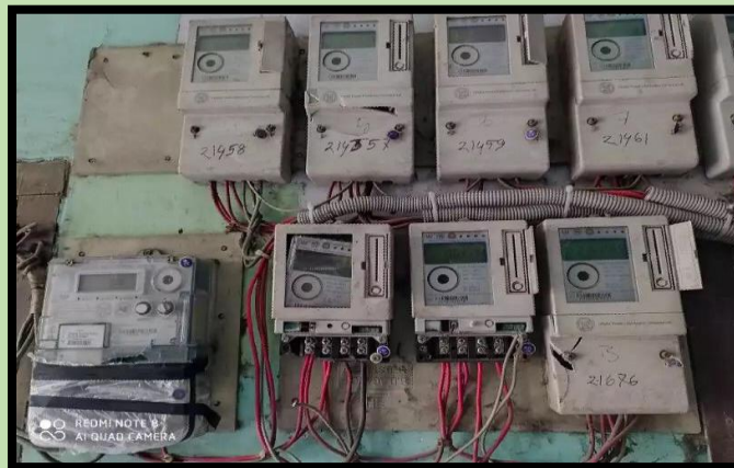
Vandalism by OST Client at Chankharpul CDIC
