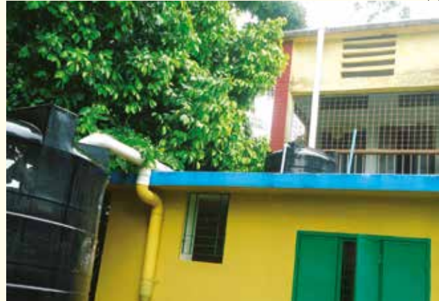
A RWH system is installed in a school building
